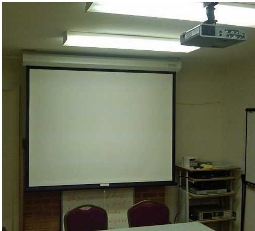
TA2 Projector Relocated to Cottage Rm 101
