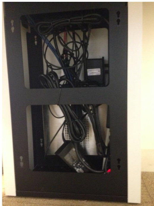
Figure 10: Example of wrong ClickShare installation: the base unit is placed inside a metallic closet without using antenna extension kit which strongly deteriorates the signal quality
