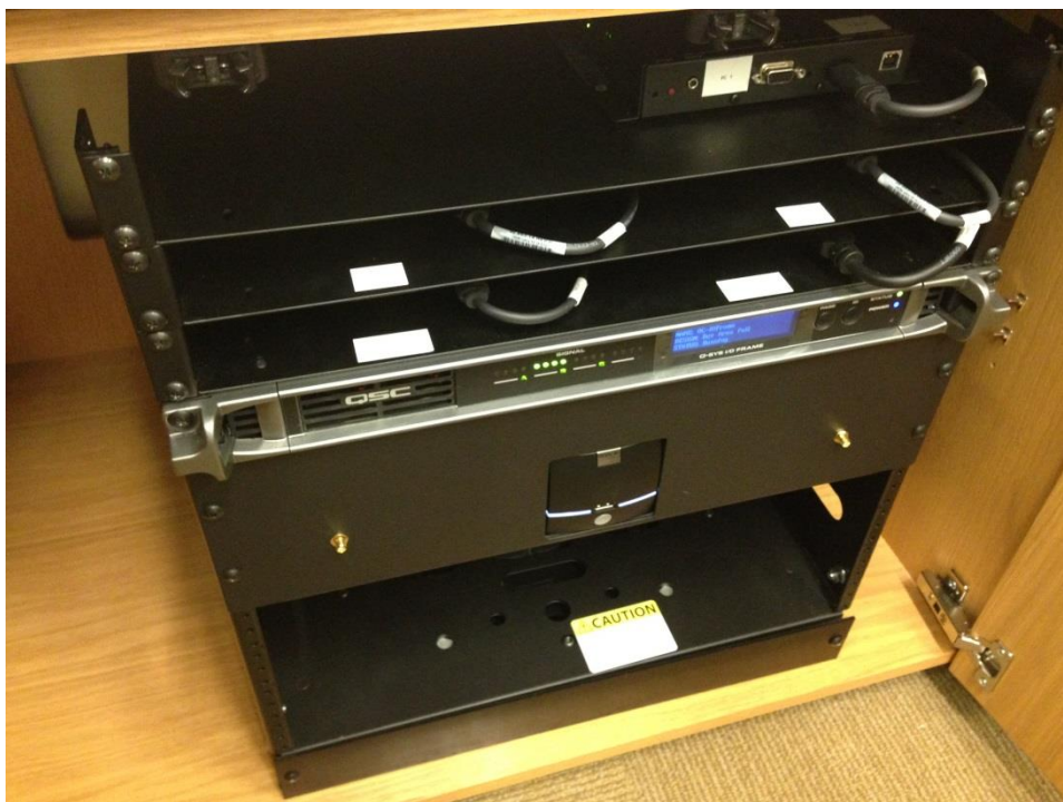
Figure 8: Example of wrong ClickShare installation: the antenna are not connected on the ClickShare rack-mounted kit
